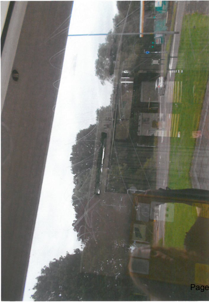
GRAFFITI on windows scratched on
