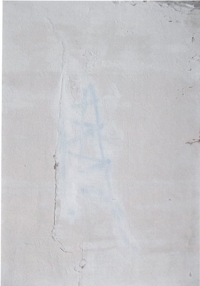
Graffiti on Back church wall
